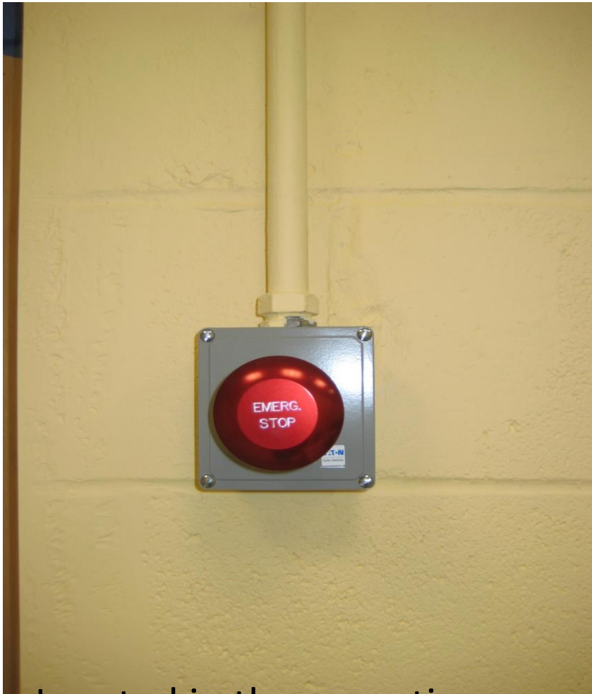
Located in the operations room
